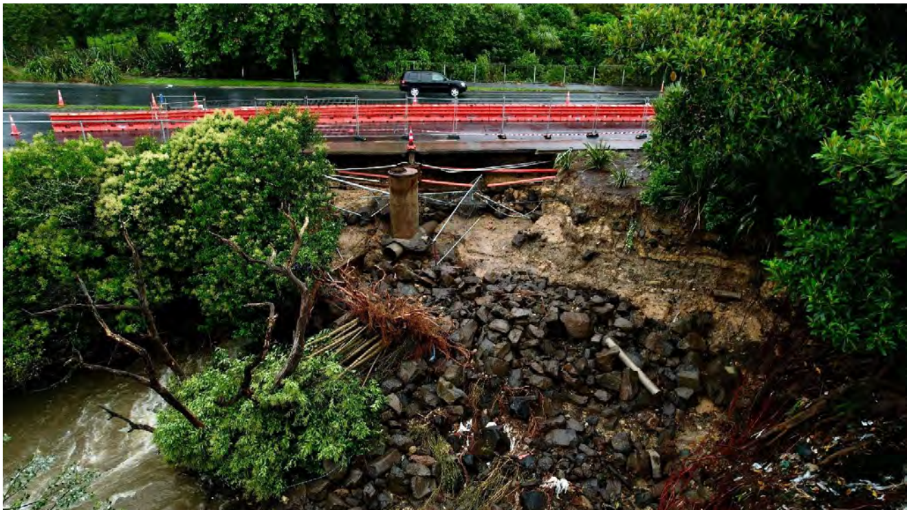
Damage to culvert on Great North Road
