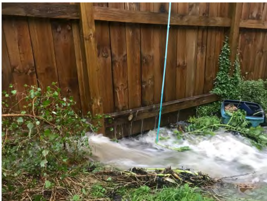
Overland flow blocked by a fence
