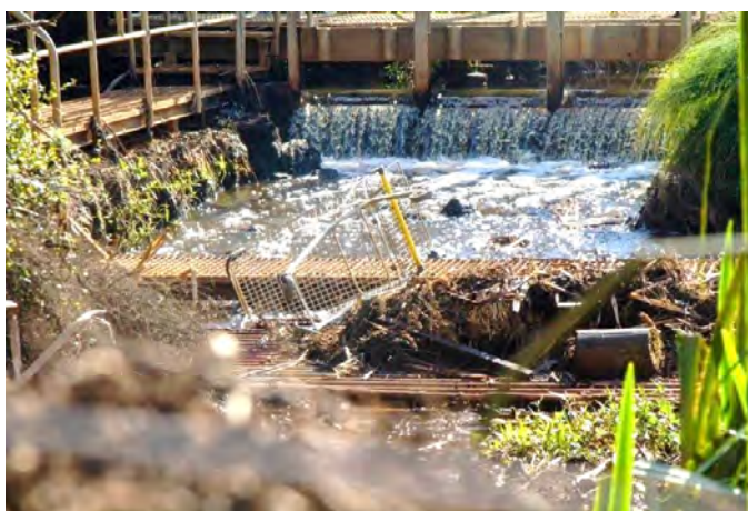
Debris and materials blocking pipe network
