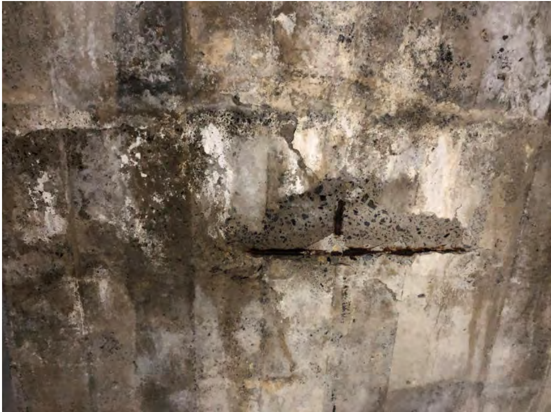
Photo 7: Exposed reinforcing with little cover
