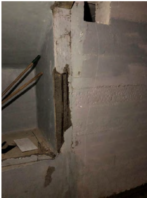
Photo 6: Spalled concrete to ammunition store
