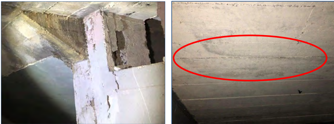
Figures 10 & 11: Storage room corridor opening & ceiling crack
