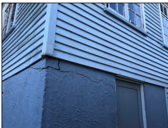
Crack in foundation wall at south corner.
