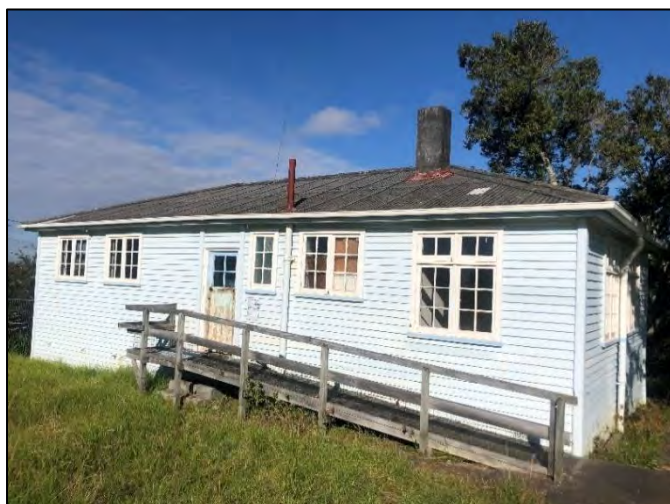
Rear side of building. Note corrugated asbestos cement roof and remnant of earlier lead flashing at the base of the chimney. Note also plastic spouting.
