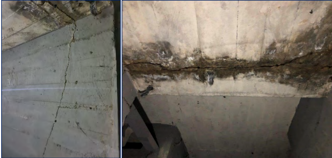
Figures 8&9: Vertical cracking around western entrance tunnel
