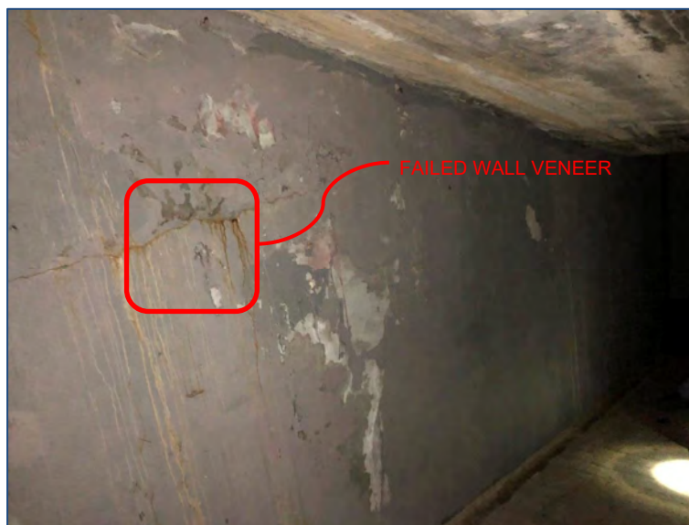
Figure 6: Southern Ramp Wall – Previous failed patch repairs
