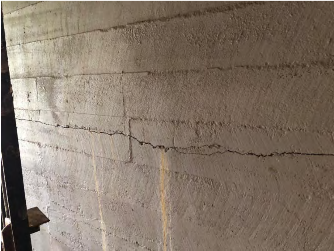
Photo 5: Horizontal crack along entire entrance wall
