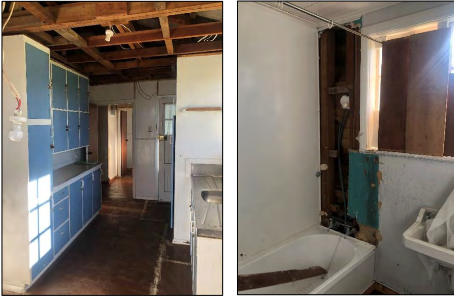
Fittings in kitchen (left) and bathroom (right).
