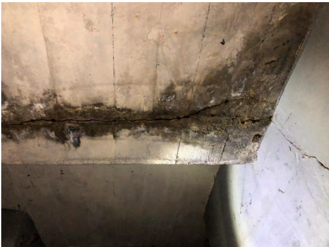
Photo 4: Large crack extending around soffit, walls and floor
