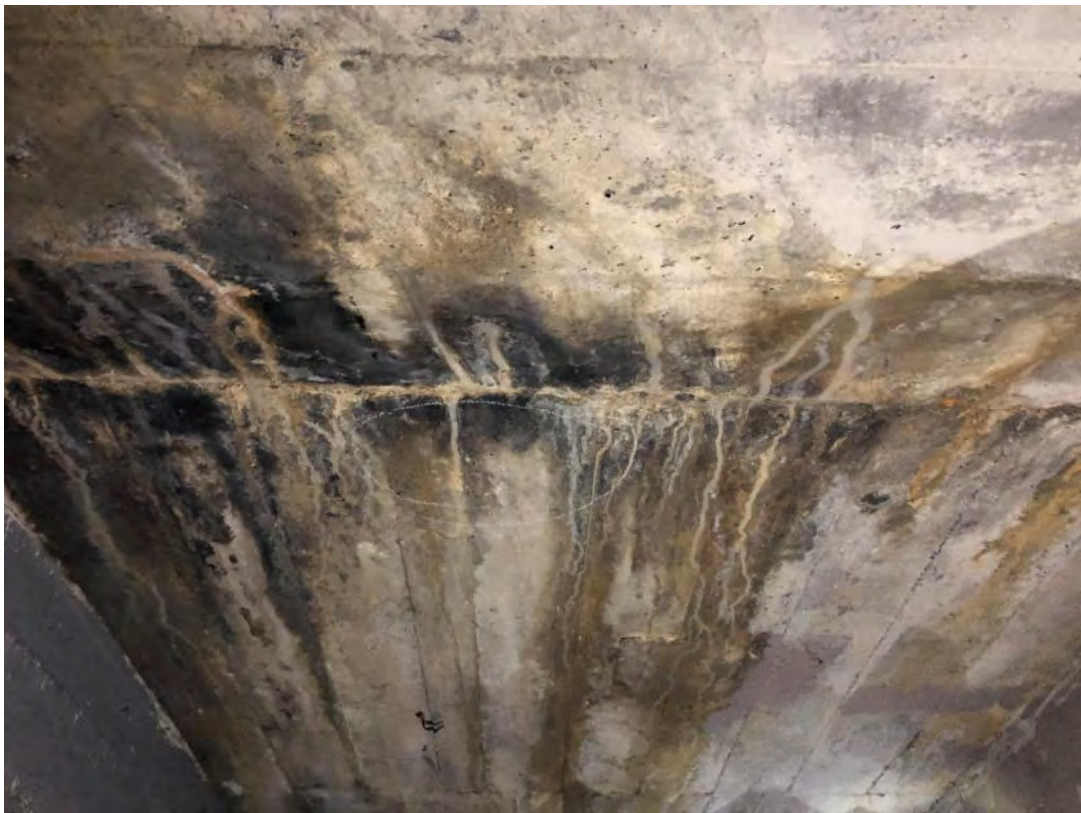
Photo 2: Water ingress and rotten concrete to soffit
