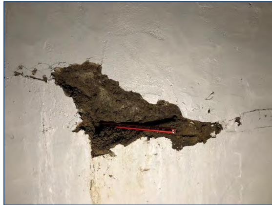
Figure 12: Damage to storage room walls
