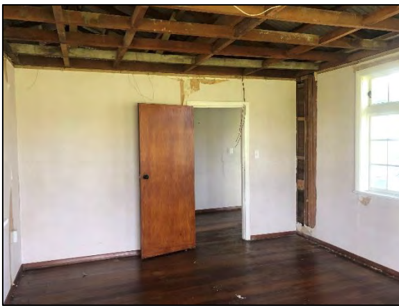
Interior of living area. Note plywood faced door and bullnose architraves and skirting.
