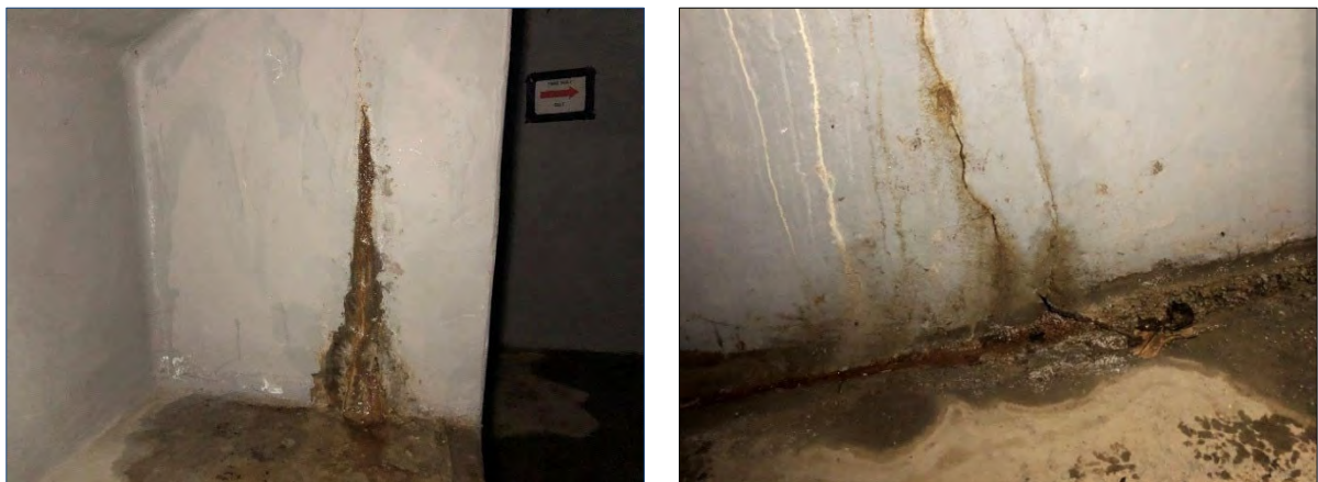
Figures 15 & 16: Corrosion staining through veneer coverings
