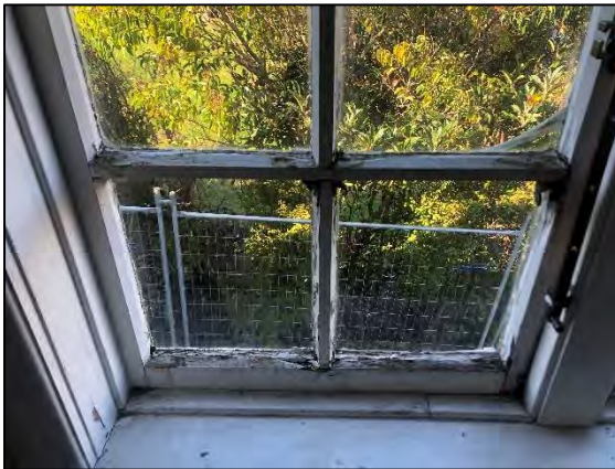
Decay apparent in replacement sash (left) and rear door (right).
