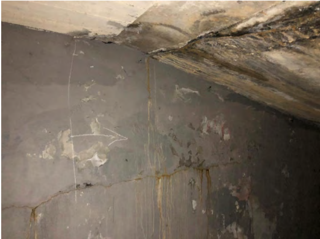
Photo 3: Failed wall repair
