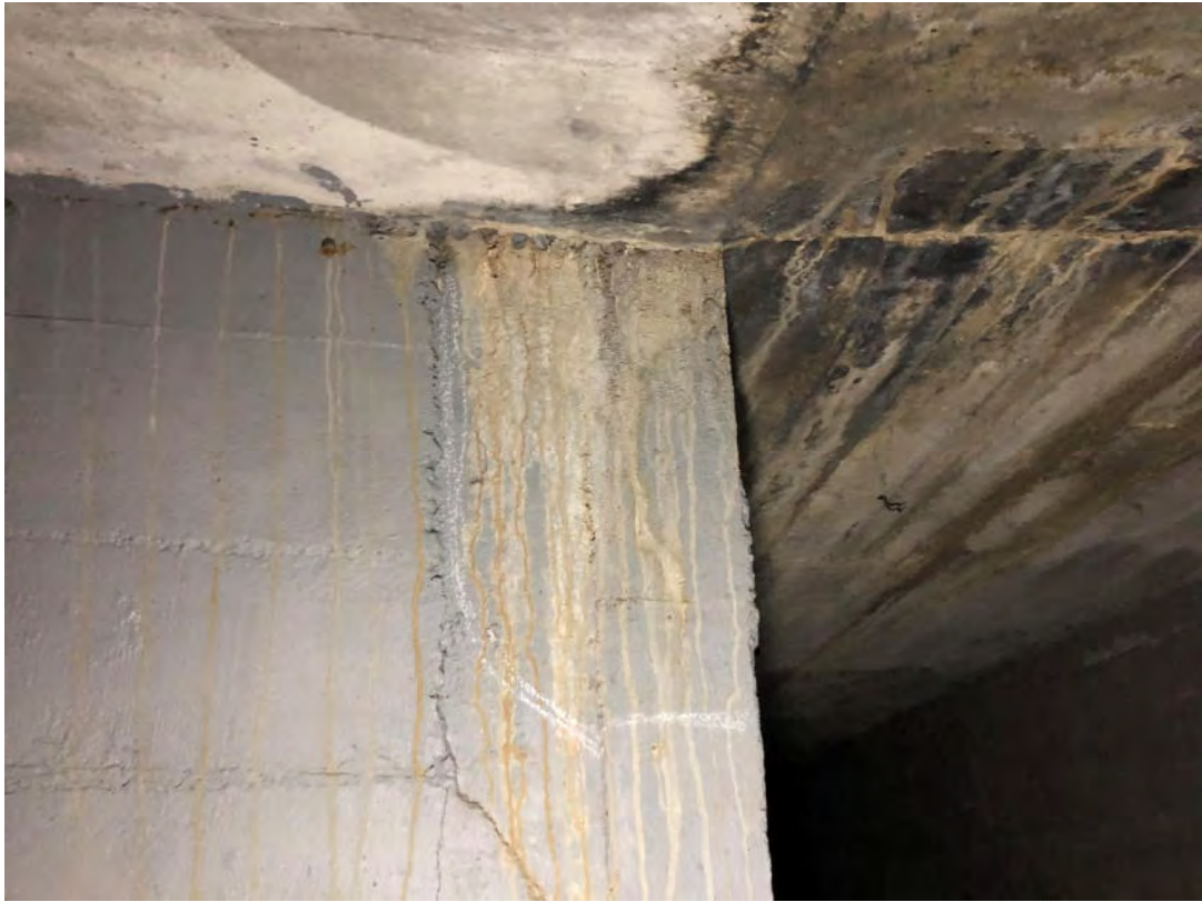
Photo 1: Rotten concrete at corner
