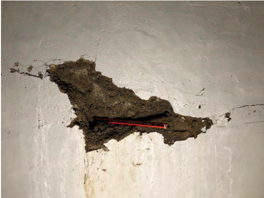
Photo 9: Rotten concrete with water seeping into service room
