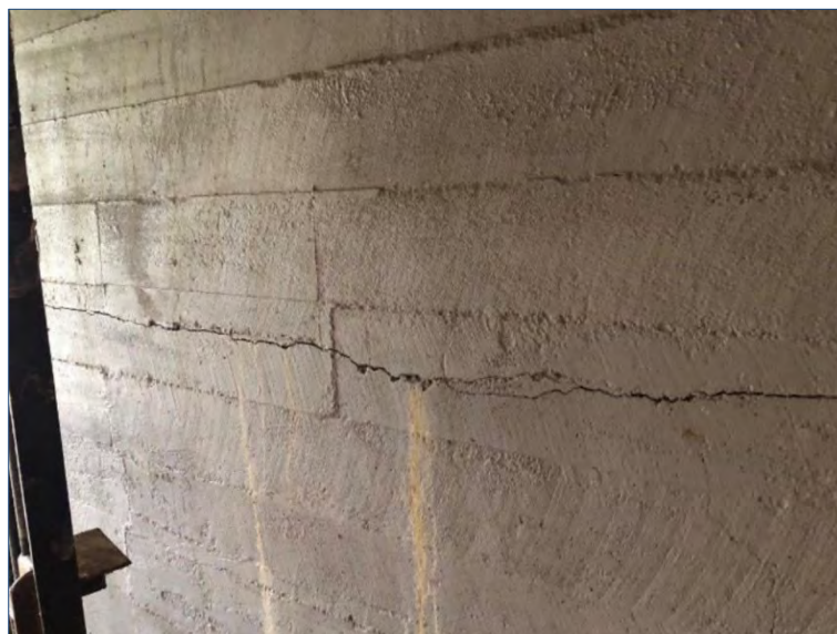
Figure 7: Horizontal cracking to western entrance tunnel
