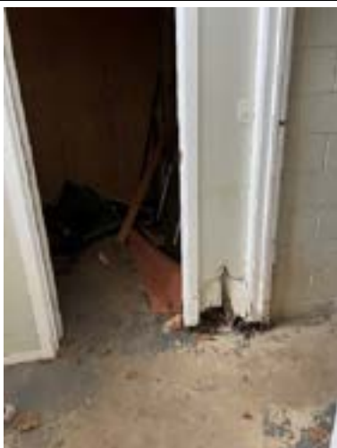
Image 4: Rotting and damaged walls throughout the building.
