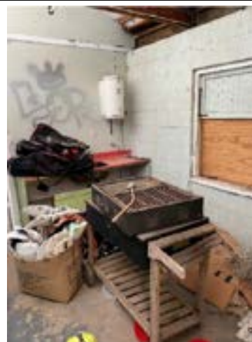
Image 5: Kitchenette area at front of building is vandalised, has poor flooring and shuttered windows.
