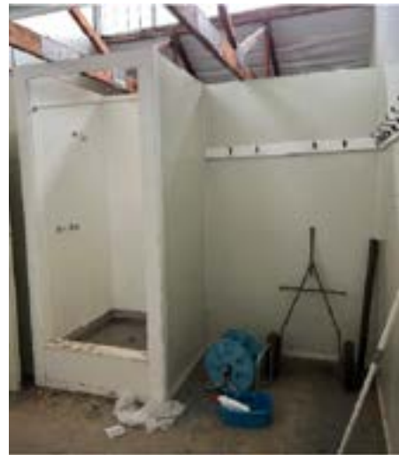
Image 3: Shower and changing area are not accessible and are in poor condition.
