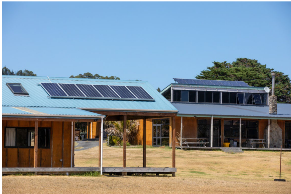
Solar panels at the Great Barrier Island Sports and Social Club
