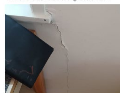
16. Cracked wall GIB board.
