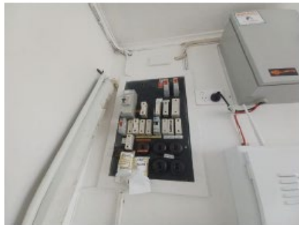
15. ACM (asbestos containing material) switchboard.
