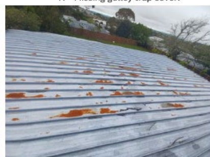
9. Rusty roof covering of toilet and kitchen area. (Addition part of the hall).
