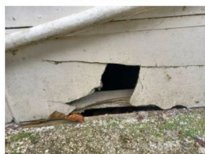
6. Damaged ACM (asbestos containing material) wall cladding.
