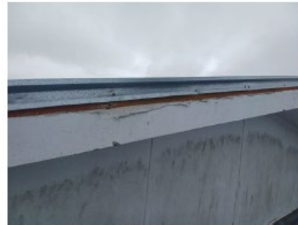
14. Loose paint on timber barge board and mould affecting gable board.
