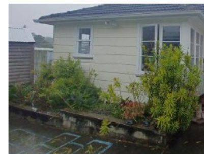
12. Garden soil level filled over cladding and gully trap.
