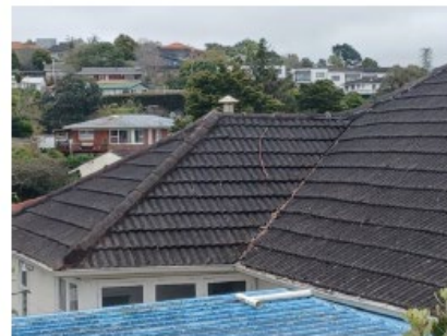
7. Very worn concrete tile roof cladding.
