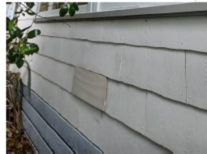
9. ACM (Asbestos Containing Material) wall cladding.
