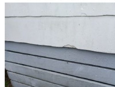
10. Cracked wall cladding.
