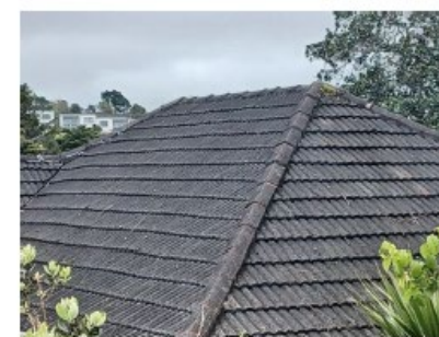
8. Poor condition concrete tile roof cladding.
