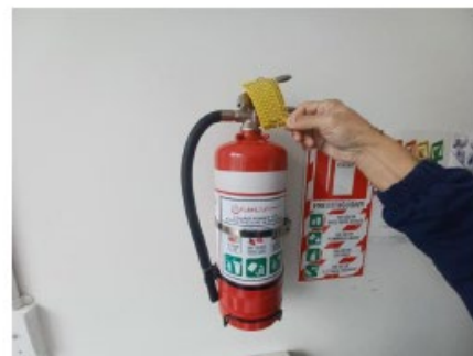
18. Expired fire extinguisher.
