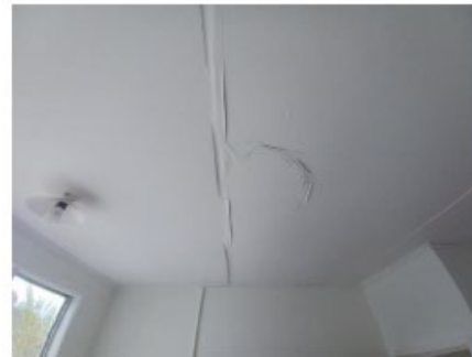
16. Cracked ceiling GIB board.
