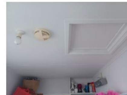
14. Smoke alarm and ceiling access hatch.
