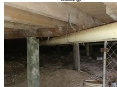
11. Piles not completely backfilled.
