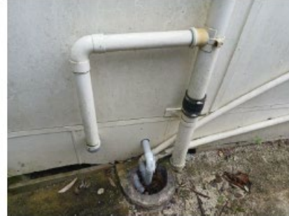
7. Missing gully trap cover.
