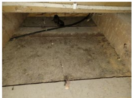
21. Views of ceiling lining in roof space. No ceiling insulation in place.
