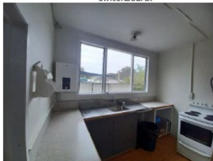
17. Rangehood not in place.
