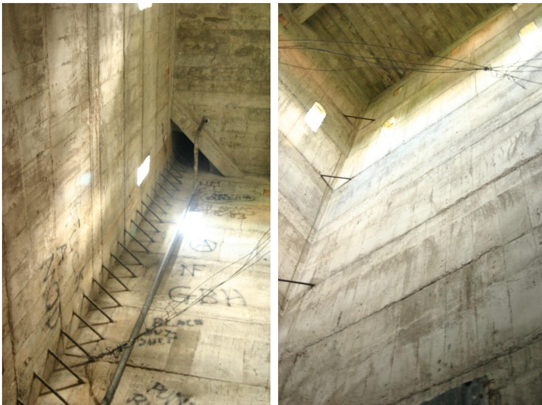
Figure 15: Views inside the tower, looking up towards the tank. Matthews & Matthews Architects Ltd 2008
