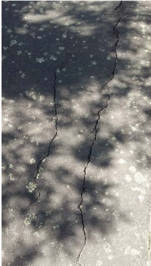
Cracked asphalt on entrance footpath
