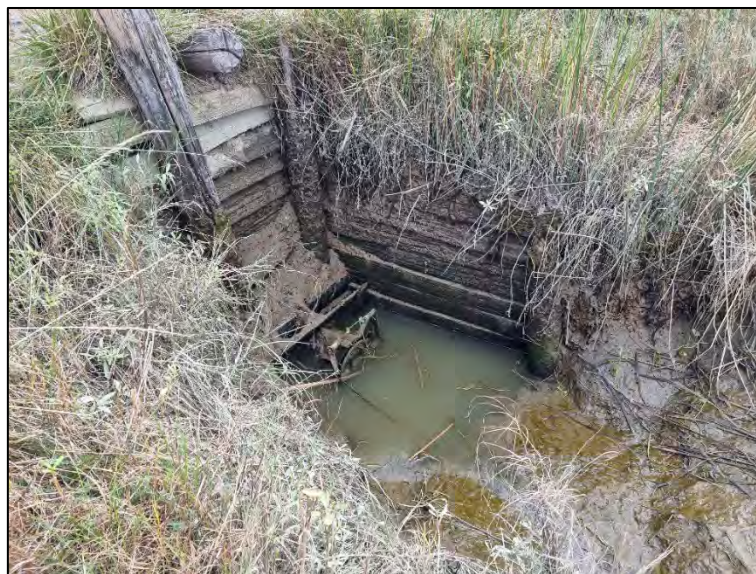
Figure 3: Flood gate outlet
