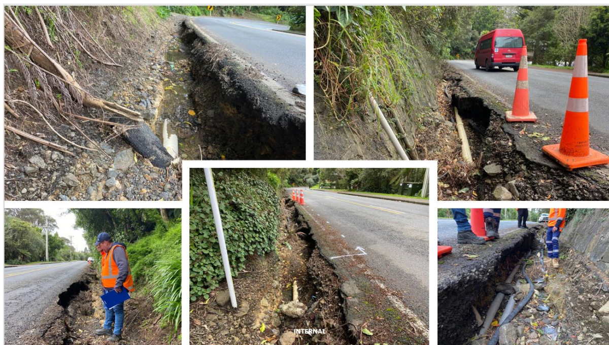
One of two Huia Rd sites with exposed services and work planned for September.
