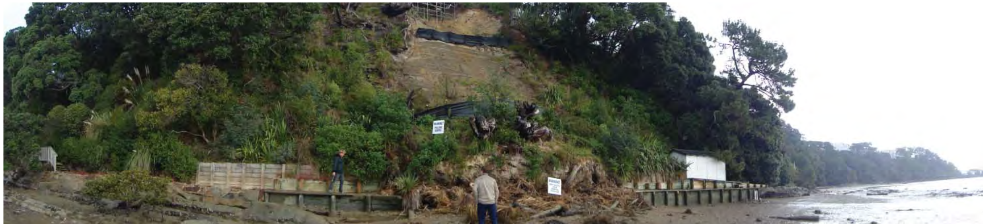
View of Hobson Bay walkway showing the slip on cliff face
