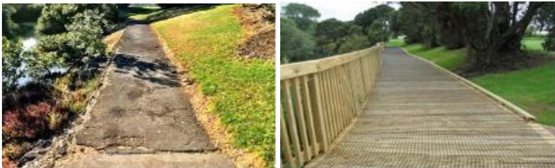
Before and after photos show the upgrade improves safety and usability of the pathways in Cox's Bay Reserve
