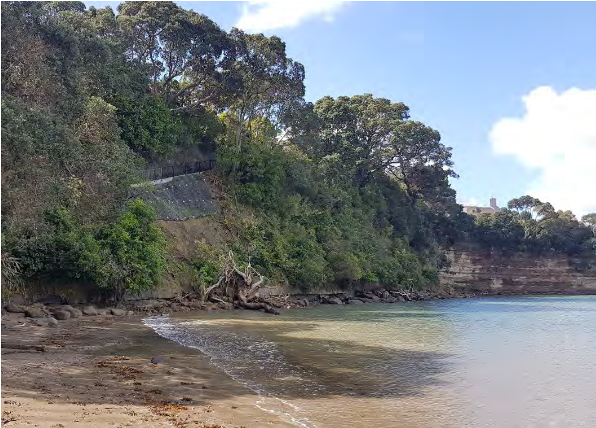
Figure 2: A typical Auckland East Coast cliff showing a recent repair to reinstate a footpath damaged by cliff instability As the toe of these cliffs is eroded, instability higher up the cliffs will increase.
