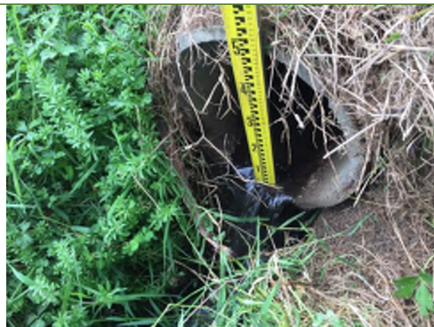
Perched undercut culvert limiting access to upstream habitat
