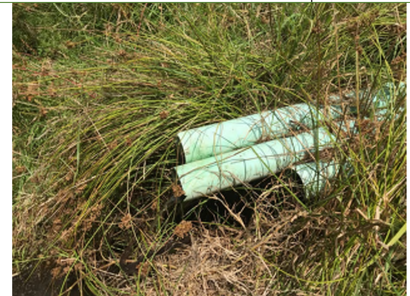
Clusters of pipes between ponds form barrier to fish passage
