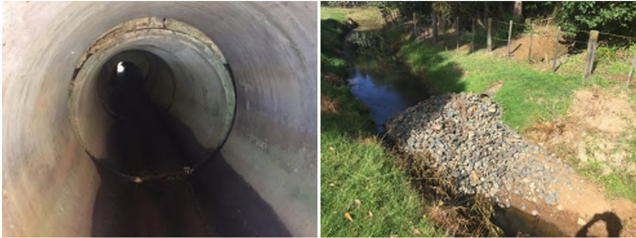
Figure 26: Left - Culvert NGAPR_044 at Great South Rd; Right - discharge of rock rip rap at Trib11_23 (NGA_155)
