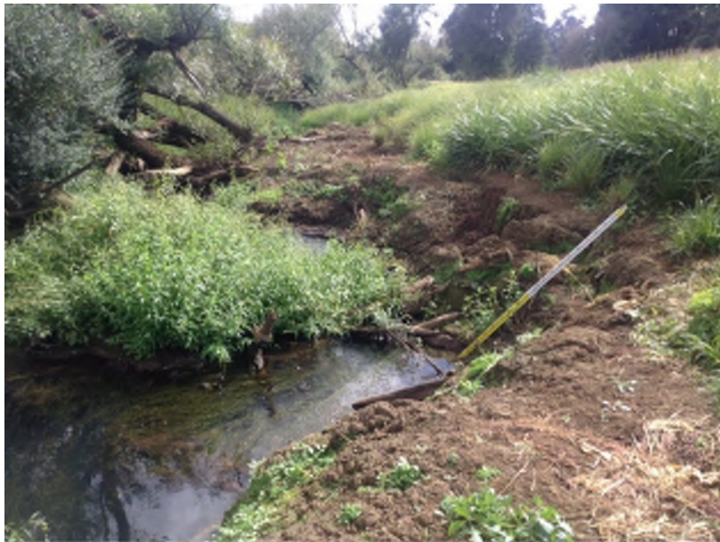
Figure 30: Erosion hotspot on NGA_MAIN_22, where slumping on the TLB has occurred as a result of poor bank vegetation and disturbance.
