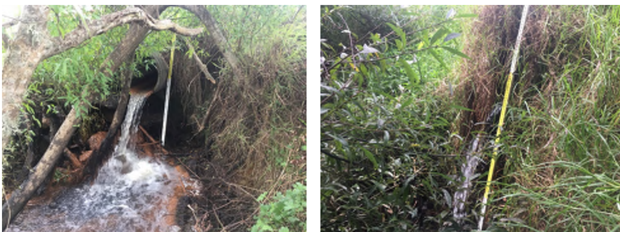
Figure 15: Perched culverts forming significant fish barriers on NGAWEST tributary. Asset ID NGAF_137 (left) and NGAF_142 (right).
