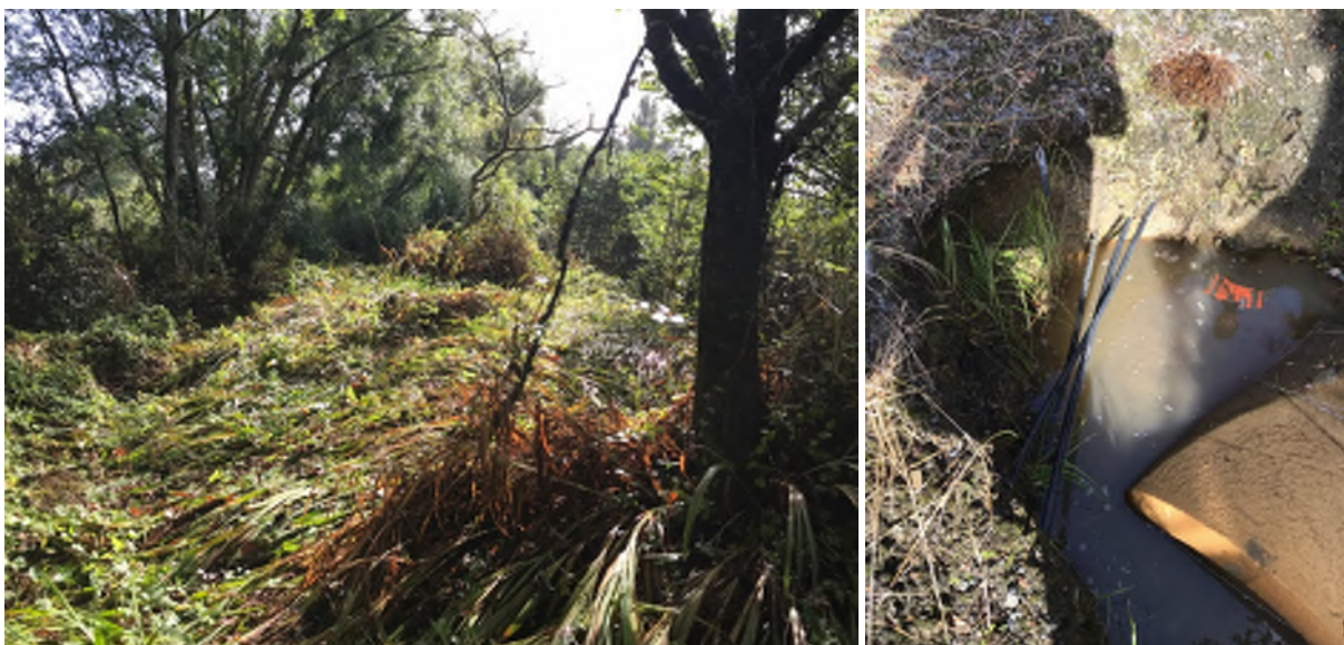
Figure 23: Left – Evidence of flooding in road corridor at Burt Rd McPherson Rd intersection. Right – Moderate erosion at outlet NGAR_074 at McPherson Rd resulting in exposed underground services
