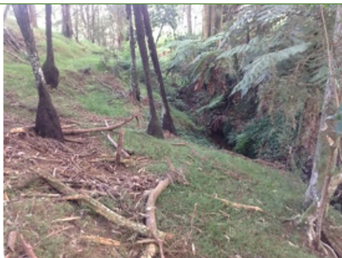
Poor density of upper bank vegetation with stability provided by existing trees
