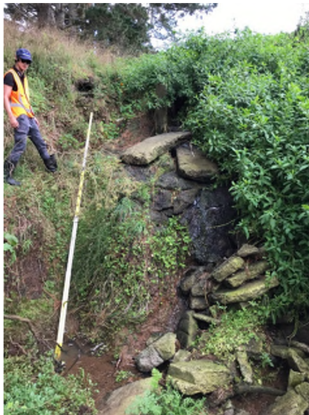
Figure 31: Culvert failure at TRIB24_6 and the associated erosion hotspot along the banks.
