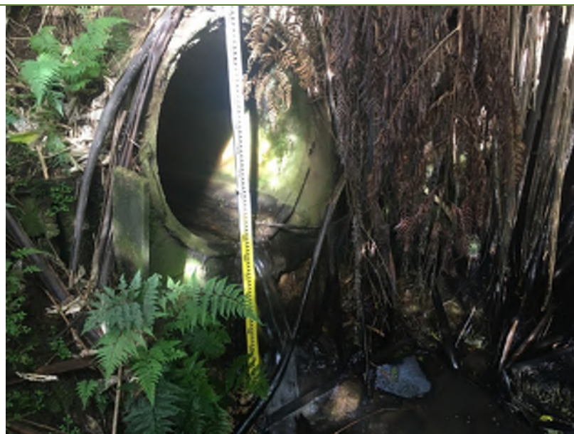
Perched culvert 0.8m above stream channel, creating a fish passage barrier (NGAF_117)
