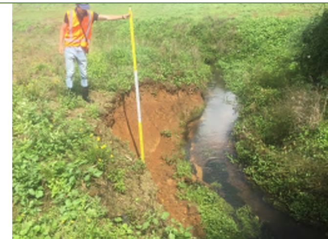
Erosion hotspot 30 m downstream of motorway outlet
