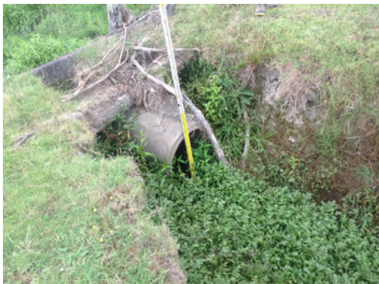
Figure 25: Erosion at outlet NGA_064 with partial collapse of retaining beams for crossing
