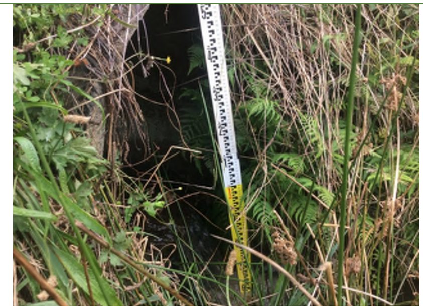
Perched culvert NGAF_130
