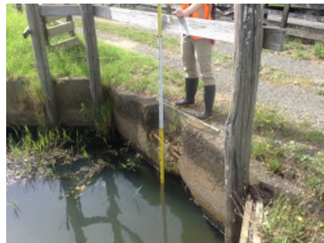
Outlet of culvert with noted flooding issues. Partially submerged.
