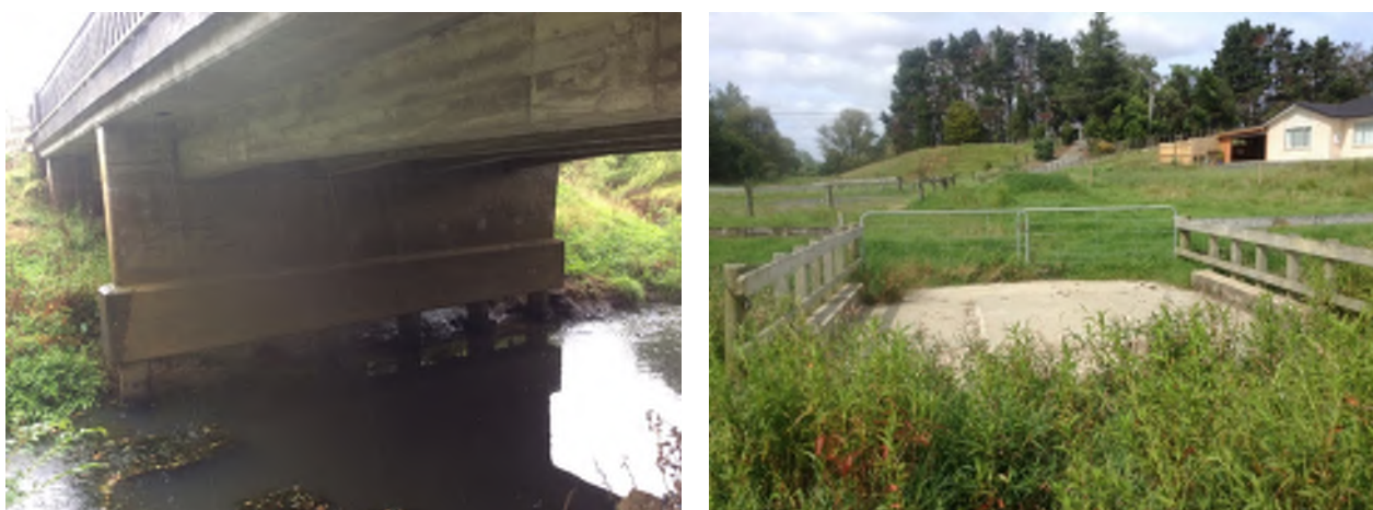
Figure 33: Bridge on Runciman Rd (TRIB9_1) with exposed piles due to scour (left). Bridge on TRIB8b_1 that poses a flooding risk (right).
