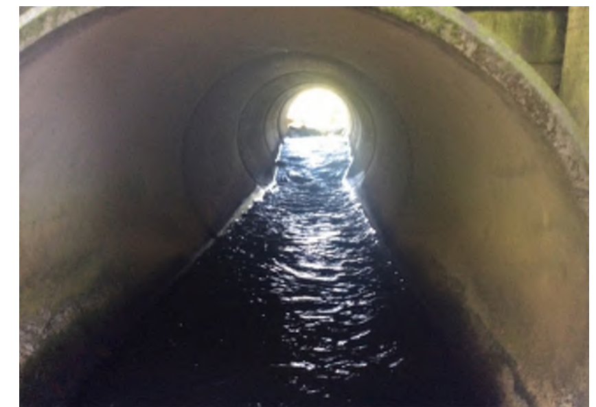
Culvert outlet showing displaced section and debris jam at inlet
