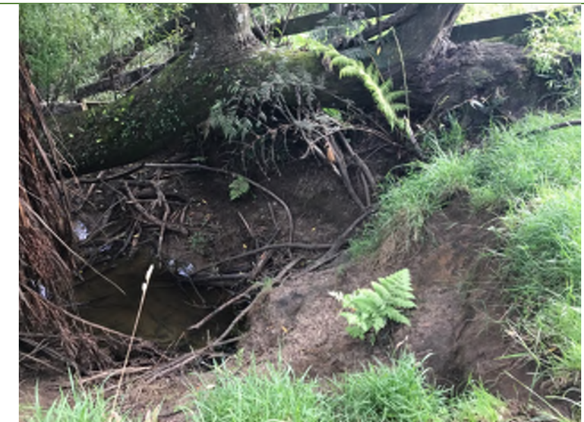
Moderate erosion at outlet from channel to main stream.
