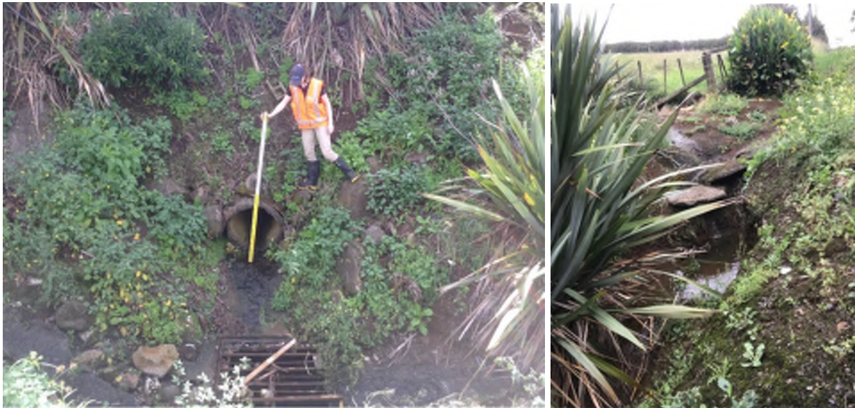
Figure 22: Left – Middle of roadside infrastructure showing pipe NGAPR_052 draining towards broken catchpit grill with inlet to Council pipe 2000200812 under this grill. Concrete reinforcing for additional outlets to the left and right. Right – facing upstream showing broken concrete dissipation.
