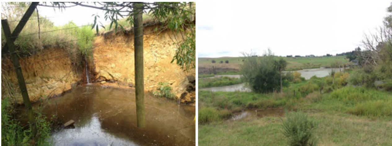
Figure 28: Dam wall breach
