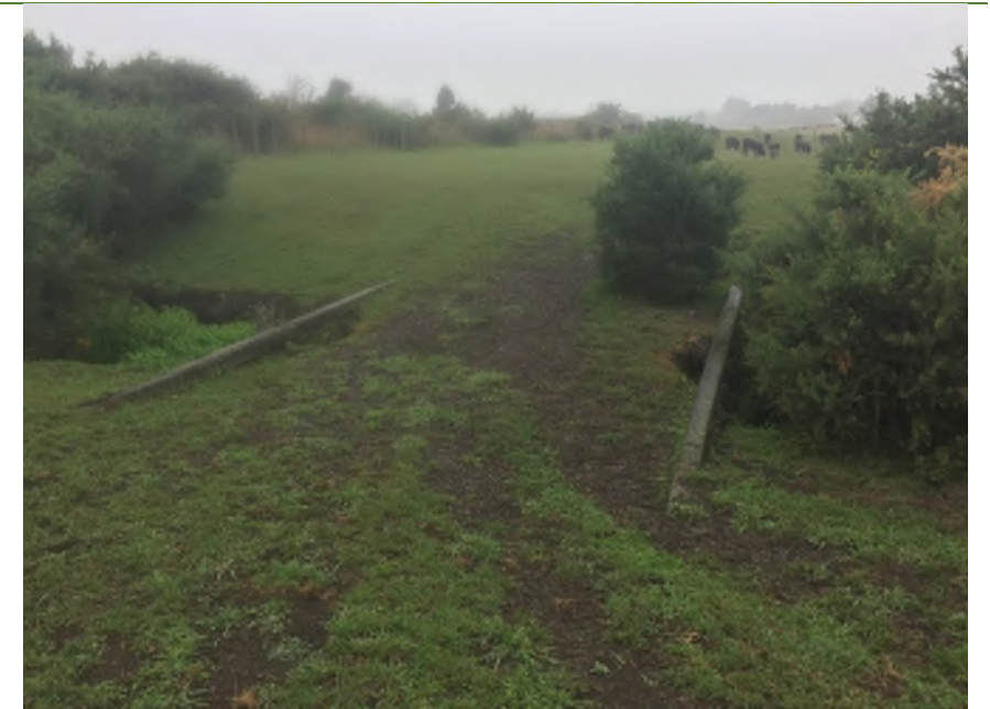
Poor condition crossing with erosion issues
