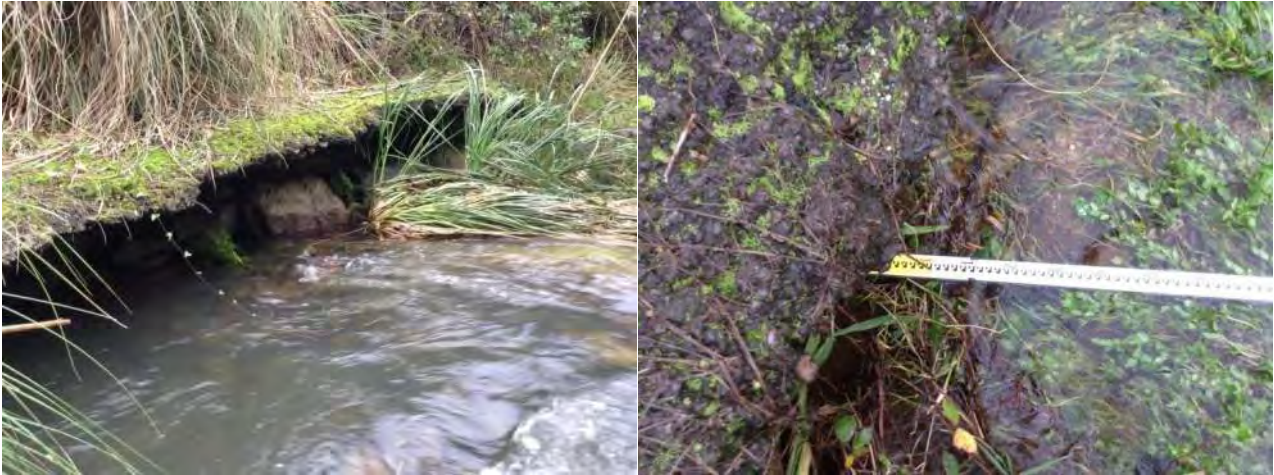
Figure 32: Undercut bank lining on HAY_MAIN_29
