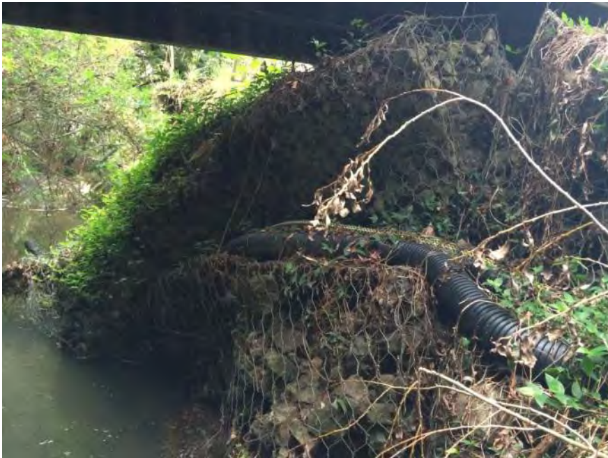
Figure 31: Poor condition bank lining on WAI_MAIN_15 under shared driveway.
