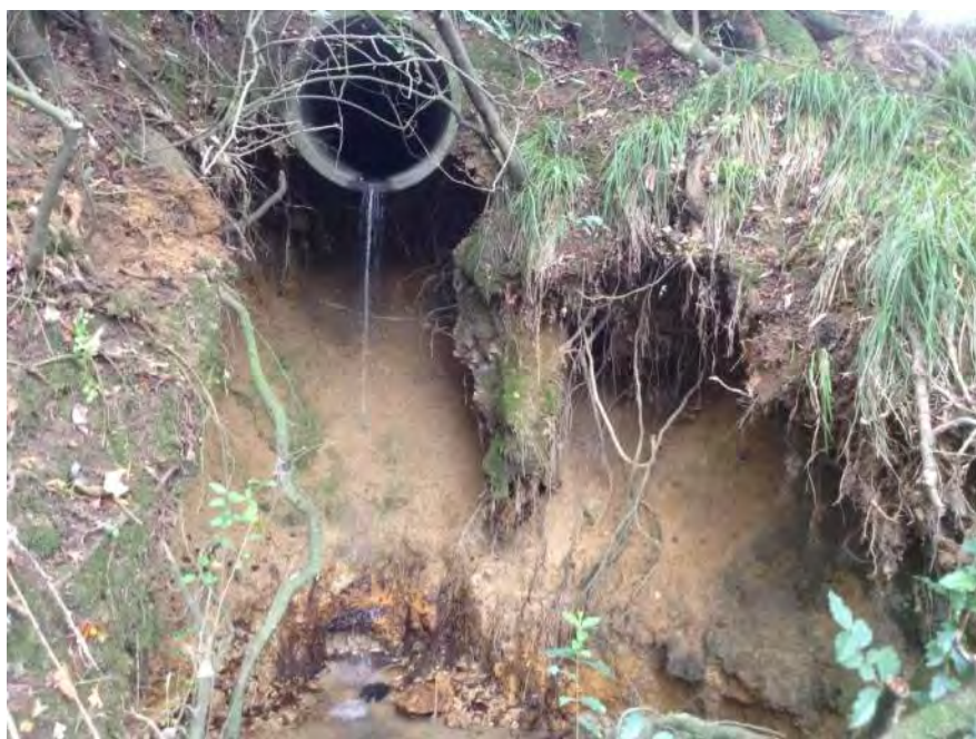
Figure 27: Severe erosion on HAY_MAIN_9 associated with asset: 1115574
