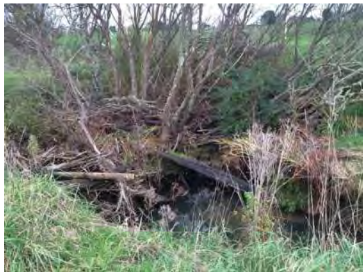
Large Willow in stream causing debris jam and obstructing flood conveyance on WAI_MAIN_9
