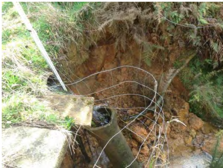
Figure 29: Severe erosion and culvert failure at HAY_TRIB6fl_2 (pond UNK_49, outlet UNK_581)
