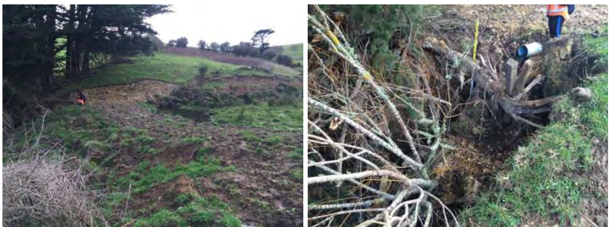
Figure 30: Recently installed culvert at HAY_TRIB6c_10 (wetland UNK_29, outlet UNK_414). A mature pine and the original concrete culvert had slipped.
