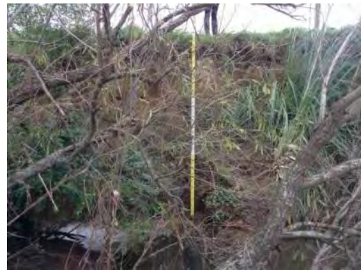
Landslip at SYM_MAIN_5
