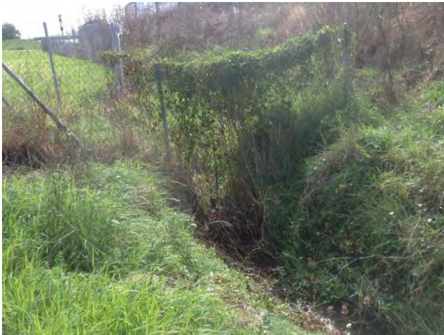
Figure 38: Wire mesh fence with debris build up potentially restricting flow on SLI_TRIB5_7
