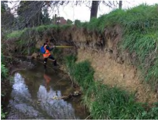
Undercut bank on true left bank on WAI_MAIN_14
