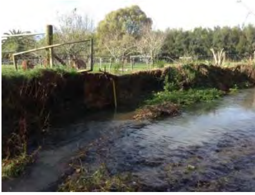
Erosion hotspot on true right bank on WAI_MAIN_10
