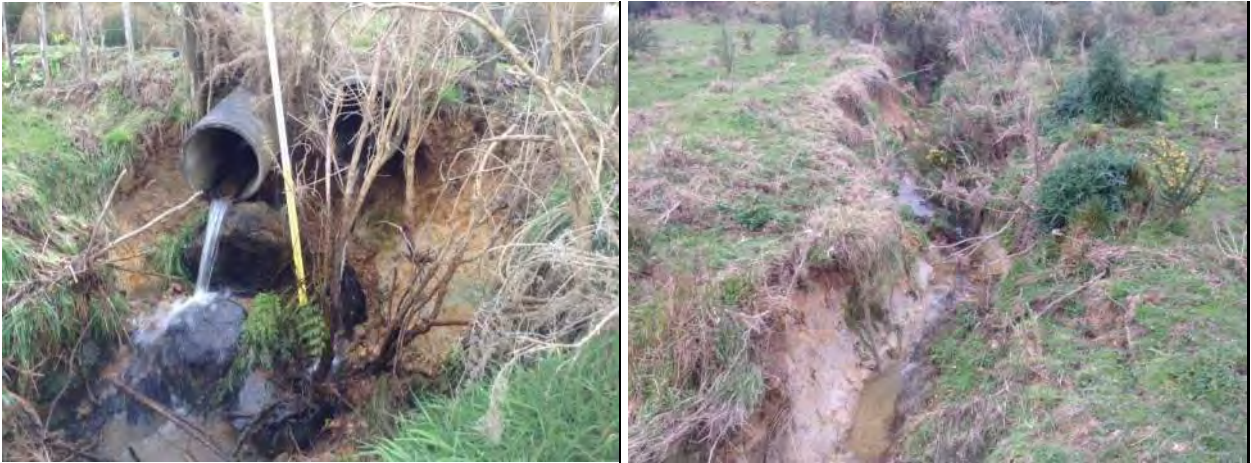
Figure 28: High velocity discharge from wetland UNK_ 117 causing severe erosion downstream (SYM_TRIB2_10) (outlets UNK_379, UNK_380)
