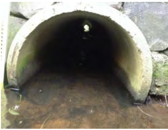
Appleby Road Drainage Improvement Project 25. Asset ID UNK_320 450mm incorrectly labelled as 900mm on project plan. Inlet ID UNK_143. Outlet ID UNK_046
