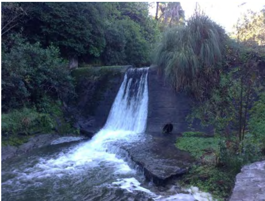
Figure 21: Old dam infrastructure at HAY_MAIN_20 with broken concrete apron
