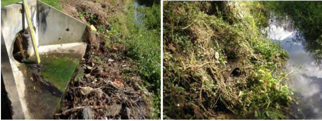
Sewage fungus at Asset 1135579. Poor condition structure separated from pipe (Asset ID 1116832)
