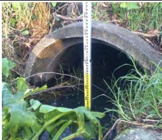
Appleby Road Drainage Improvement Project 25. Asset ID UNK_288. Inlet UNK_218. Outlet UNK_184
