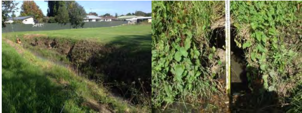
SLI_TRIB5a_1 install course sediment trap (Asset ID 1115109). Greenhaven Water Quality Management ICMP Project 21
