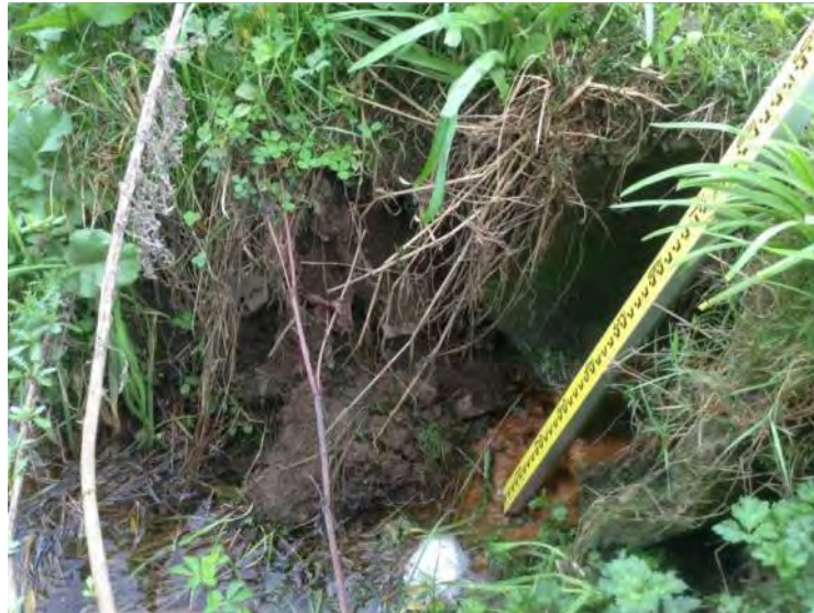
Erosion protection and structural repair required at outlet Asset ID 1115547
