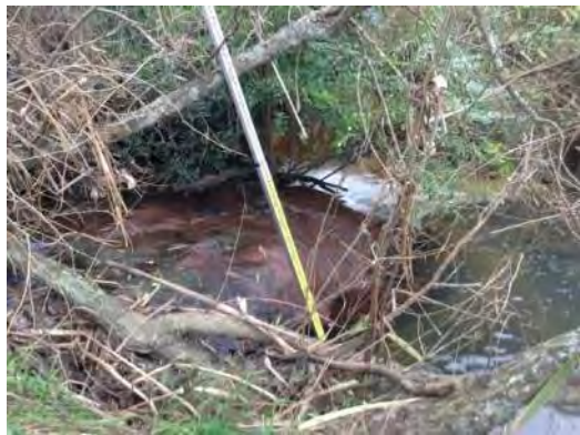
Cascade over Willow roots. Scoured pool immediately downstream with bank slip at SYM_MAIN_5
