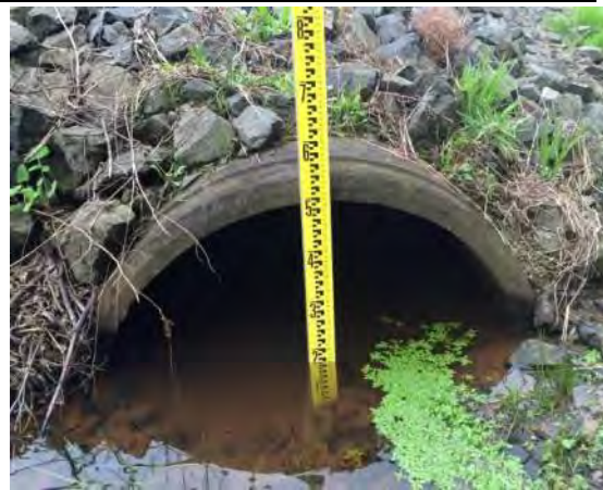
Appleby Road Drainage Improvement Project 25. Asset ID UNK_282. Inlet UNK_186. Outlet UNK_185
