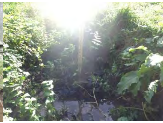
Appleby Road Drainage Improvement Project 25. Asset ID UNK_321. Inlet UNK_045. Outlet UNK_042
