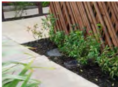
Service covers located in 600mm strip in front of fence, planting to screen.
