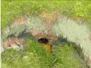
WS1 C, showing catchment and a collapsed tile drain (also found at site A and B).
