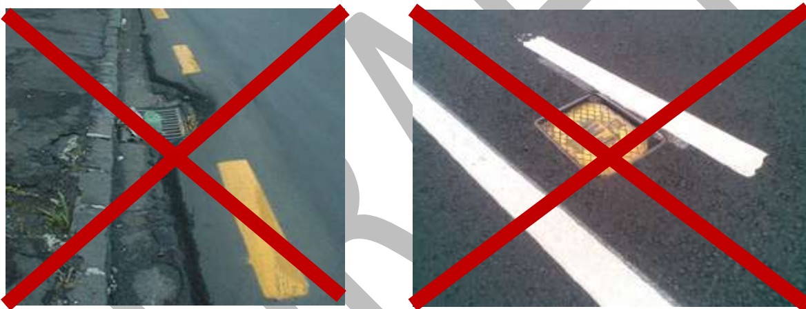
Figure 42: Examples of maintenance issues, creating hazards to cyclists – through high asphalt lips at road edge (left) and sunken cover (right)
