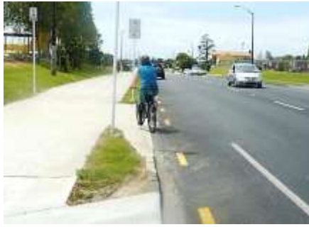
Figure 37: Example of transition between cycle lane and shared path (Central Park Drive AKI)
