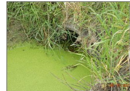
CULVERT: POOR FLOW
