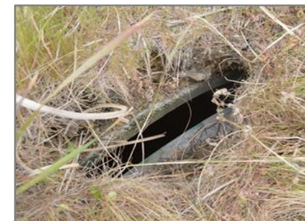
CULVERT: STRUCTURAL FAILURE
