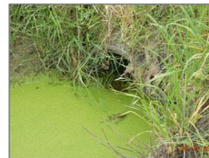
CULVERT: POOR FLOW
