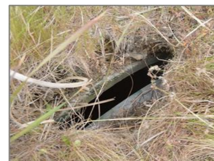
CULVERT: STRUCTURAL FAILURE
